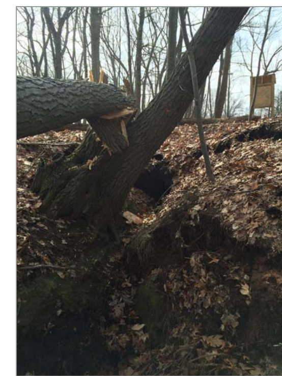
Erosion at Outlet 4/13/15 Photo 4
