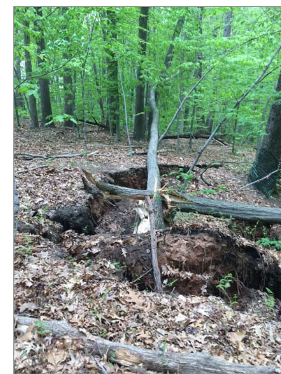
Sloughing at Outlet 5/11/15 Photo 3
